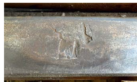
Rys. 5. Wada sguat szyny, oznaczenie 227 Fig. 5. Defect rail sguat, designation 227
